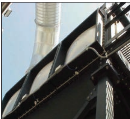
FIGURE 4. The photo shows explosion venting of a dust collector. A vented flameball is a mass of dust and combustion gases over 2,000°F that may extend 30–100 ft from the point of exit. Simple free venting must be to a safe location where personnel will not be present and other equipment cannot be damaged
